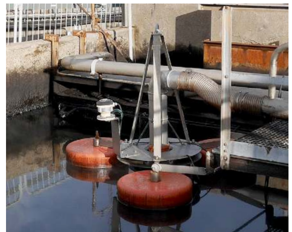
An Ultra-SurfCleaner operating in an API separator.
